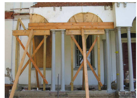
Temporary support of the arches, roof and central tower was provided during restoration.
